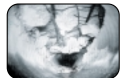
Collapsed concrete stormwater line beneath a process facility
